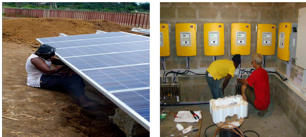
Figure 17b - Kpandebu Growth Centre 16 kW PV system in commissioning
