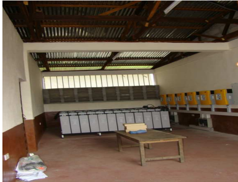
Figure 11 - Bo battery house in training area
